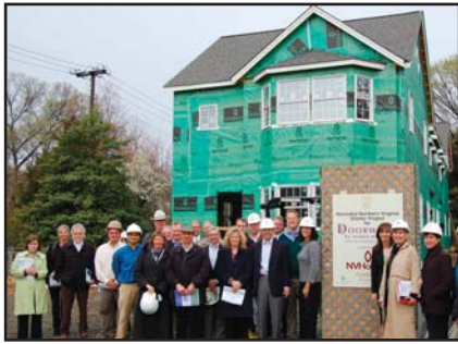
Builder Captain NVHomes hosted a hard hat tour of the new Doorways shelter in Arlington for the Board members of HomeAid Northern Virginia and other guests.
